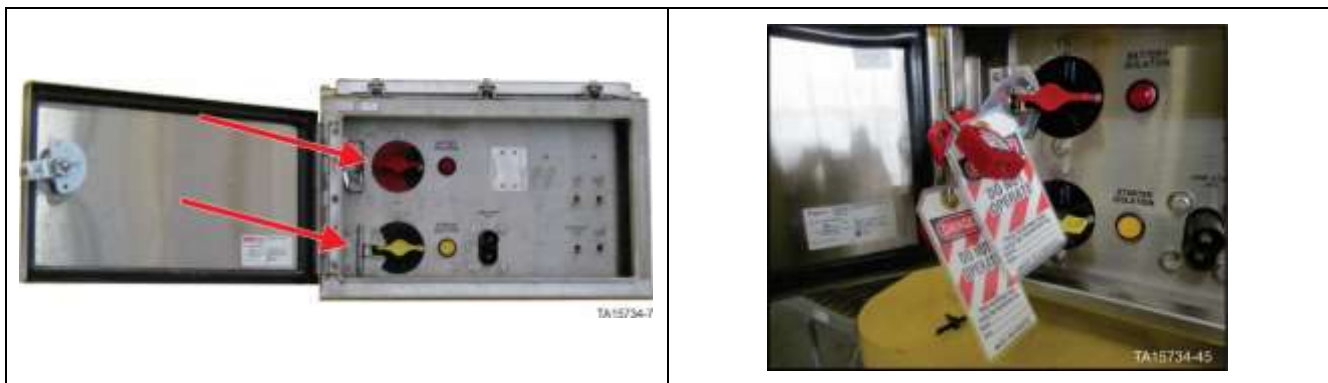
Figure 9. GEN 2 Battery Isolation Box – Battery isolation switch in OFF position with locks in place
