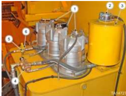
1) Return Filter Housings, 2) Relief Valve, 3) Surge Reservoir, 4) Automatic Air Release Valve, 5) Manual Reservoir Vent Valve, 6) Filler Cap
