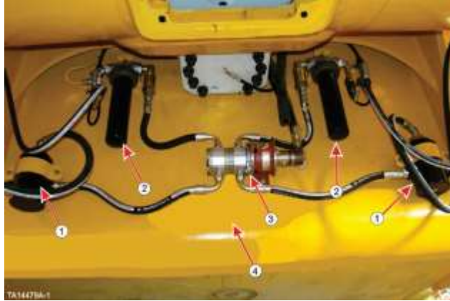
1. Rear Strainer (2) 1 For Each Planetary Drive), 2) Rear Canister Filter (2) (1) For Each Planetary Drive), 3) Pump/Motor (2) (1 Rear, 1 Inside Front Frame), 4) Fuel Reservoir (1)
