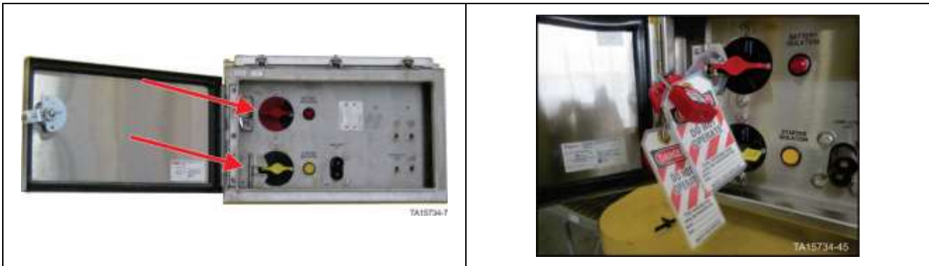
Figure 13. GEN 2 Battery Isolation Box – Battery isolation switch in OFF position with locks in place
