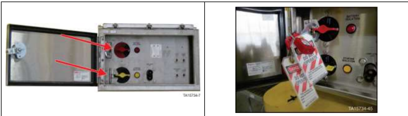
Figure 29. GEN 2 Battery Isolation Box – Battery isolation switch in OFF position with locks in place
